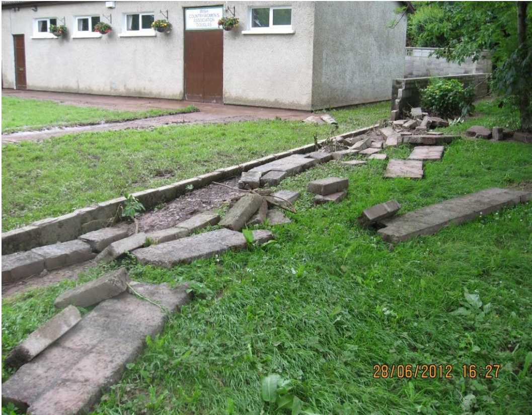
Figure 2.6: Post 2012 flood event – wall knocked down outside ICA Hall
